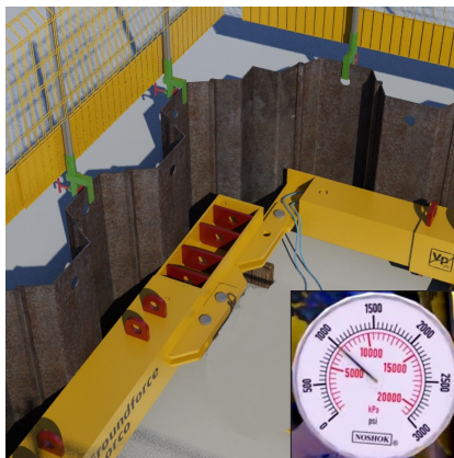
13. With all legs now connected, open the lock off valve and pressurise the brace against the trench sheets to approximately 1000psi (~70bar # ) unless otherwise stated.
